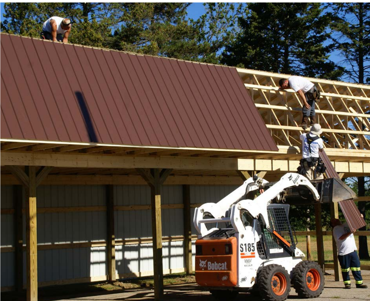
Members of VFW Post 3769 in Pikeville, Ky., and contractors build the roof of the VFW National Home for Children's new carport in June. The carport will help extend the life of the National Home's fleet vehicles during the summer and winter months in Michigan. PHOTOS COURTESY OF VFW NATIONAL HOME FOR CHILDREN
