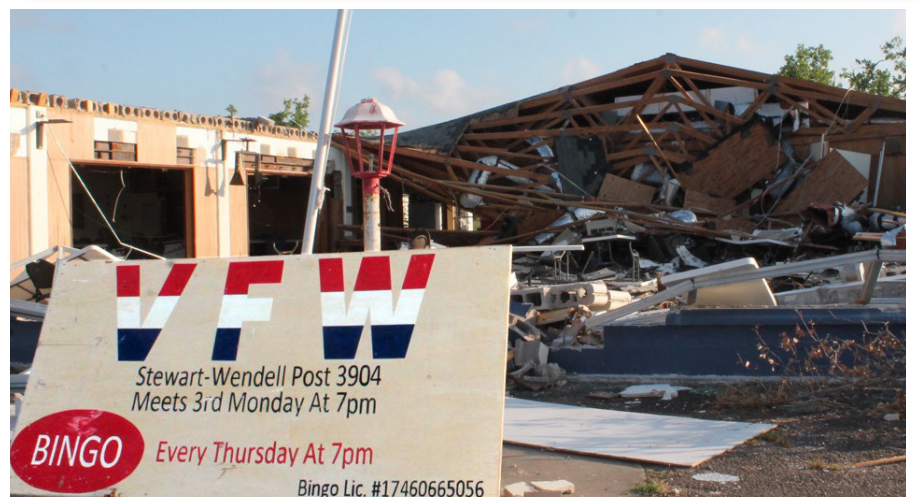
When Hurricane Harvey made its way through Rockport, Texas, winds blew in the front windows of VFW Post 3904, air pressure caused the roof to separate from the building and part of the front wall fell in, according to Post Commander Jimmy McCombs. Despite the destruction of the Post, its members met in the parking lot, surrounded by the debris, in their first meeting after the storms.
